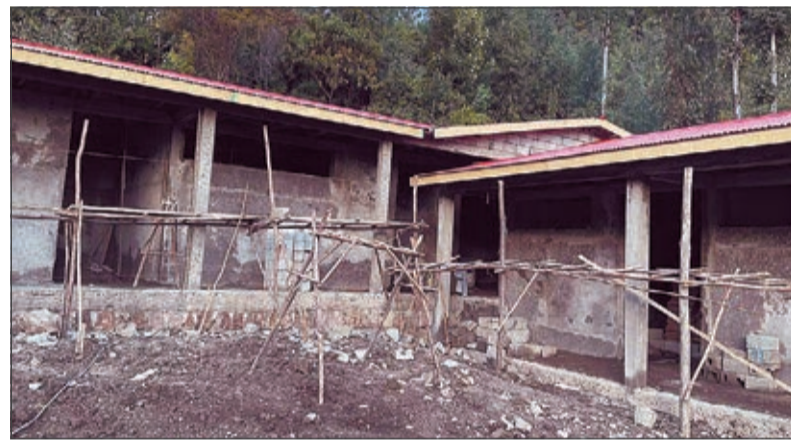
Shown above is part of the vocational center that is under construction. This center will train young people in the trades of woodworking, metalworking, hair dressing and tailoring.
