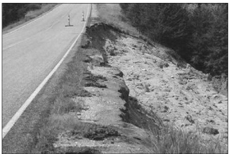
This is Lake Alvin on the east side of the lake across from the from the spillway. This road is closed because of the dangerous washout of the road. The whole big bank of dirt is completely washed away down into 9 mile creek.
