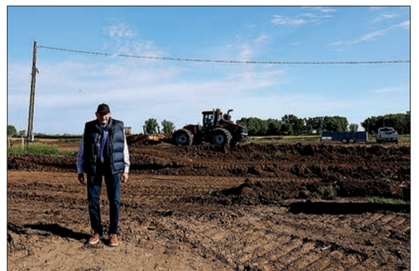
Lincoln County Commissioner Jim Jibben shows the dirt work has begun on West Street for the new Justice Center. The land will be leveled off to prepare for the building. "Luckily no trees or major issues have come into factor," added Jibben. "I am excited to see this project being started."
