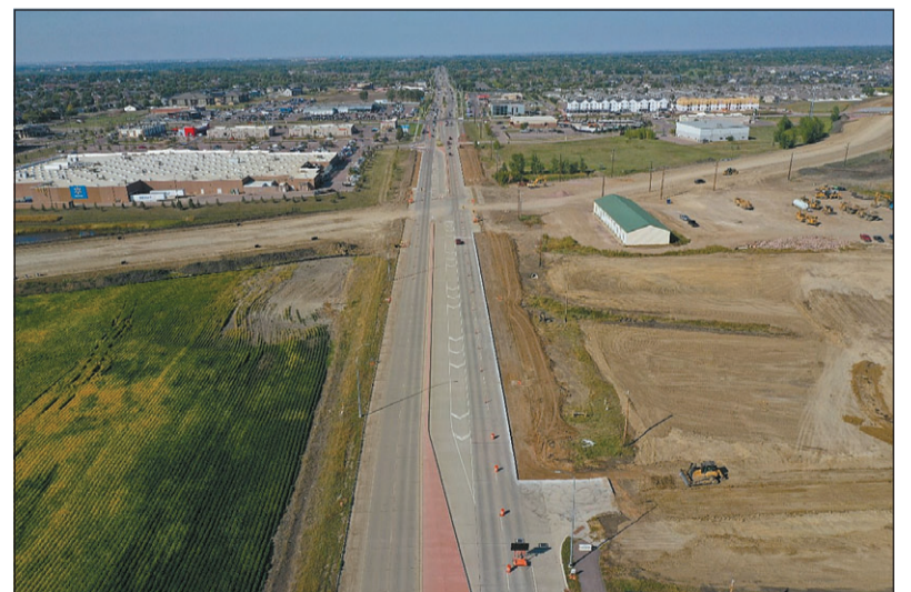
An aerial view of the South Veterans Parkway project looking north on Minnesota Avenue. Walmart is pictured to the left. Photo by Infrastructure Design Group
