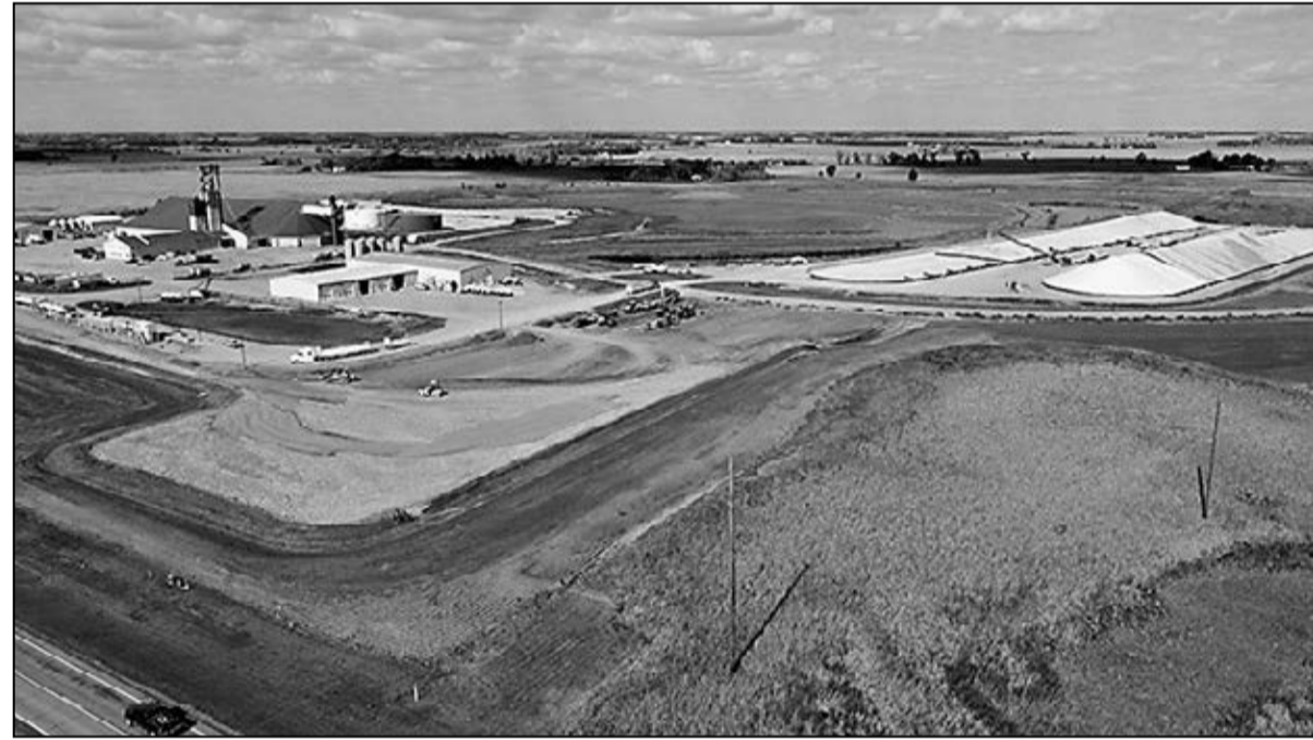
Dirt work has begun at the future site of the CHS grain shuttle facility in Worthing, South Dakota.
